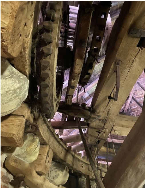
Drive to turn the mill cap
